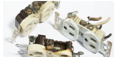
Damaged Electrical Outlets
